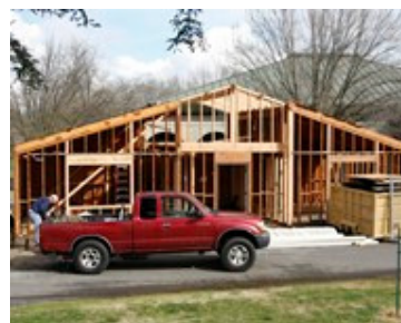
The Davis Clubhouse was taken down to the studs during the renovation.
